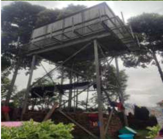
Figure 1: Tinga Ekoru Water Project Ekoru
